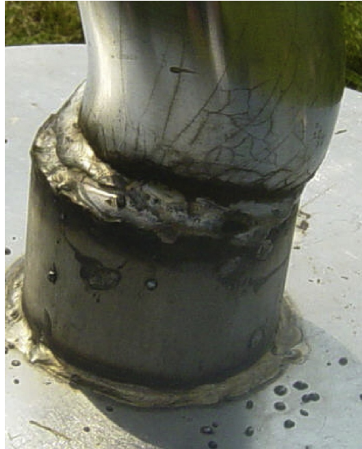
Fig. 1.13 Stress corrosion cracking of austenitic stainless steel [40]. http://www.metallurgicalviability.com/SCC.htm .
