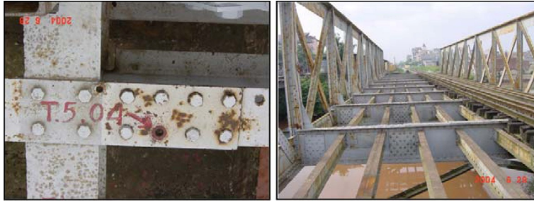
Fig. 1.4 Atmospheric corrosion of a railway bridge in Vietnam [17].
