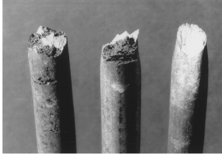
Fig. 9.50 Fracture surface of broken hanger of dead concrete roof, made from stainless steel [181].
