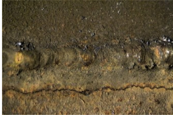
Fig. 1.15 Stress corrosion cracking near the weld of heating pipes [44].
