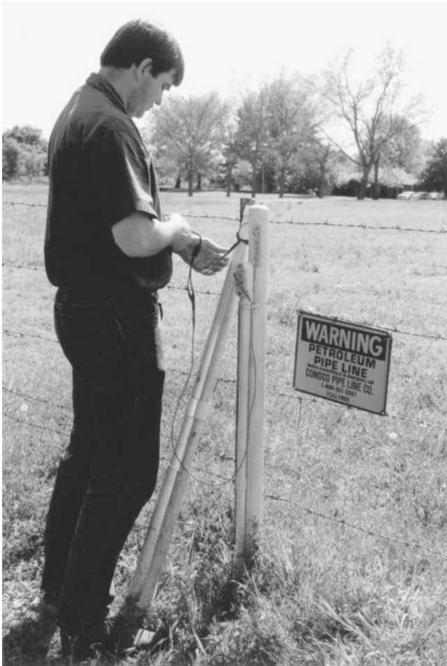
Figure 11.21 Test station with an electrical connection to the pipeline. (Courtesy of CSIR North America Inc.)
