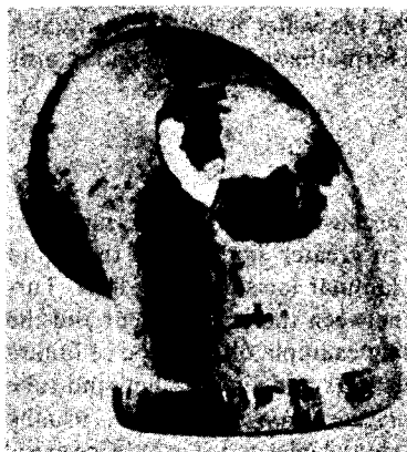
Figure 3-45 Impingement failure of elbow in steam condensate line.
